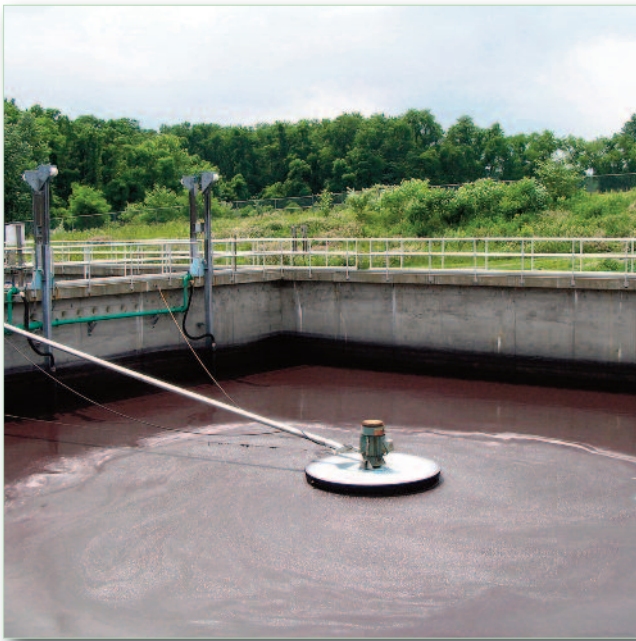
Lycoming County Water and Sewer Authority's wastewater treatment plant. Credit: Megan Lehman
