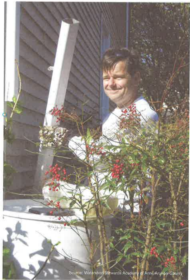
A master watershed steward installs a rain barrel at a residential property to slow the flow of stormwater runoff.
