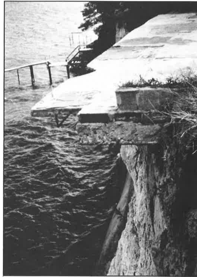
Figure 25. Erosion of the Western Shore cliffs has resulted in loss of houses (Randle Cliffs area) (photo by Stephen Leatherman).
