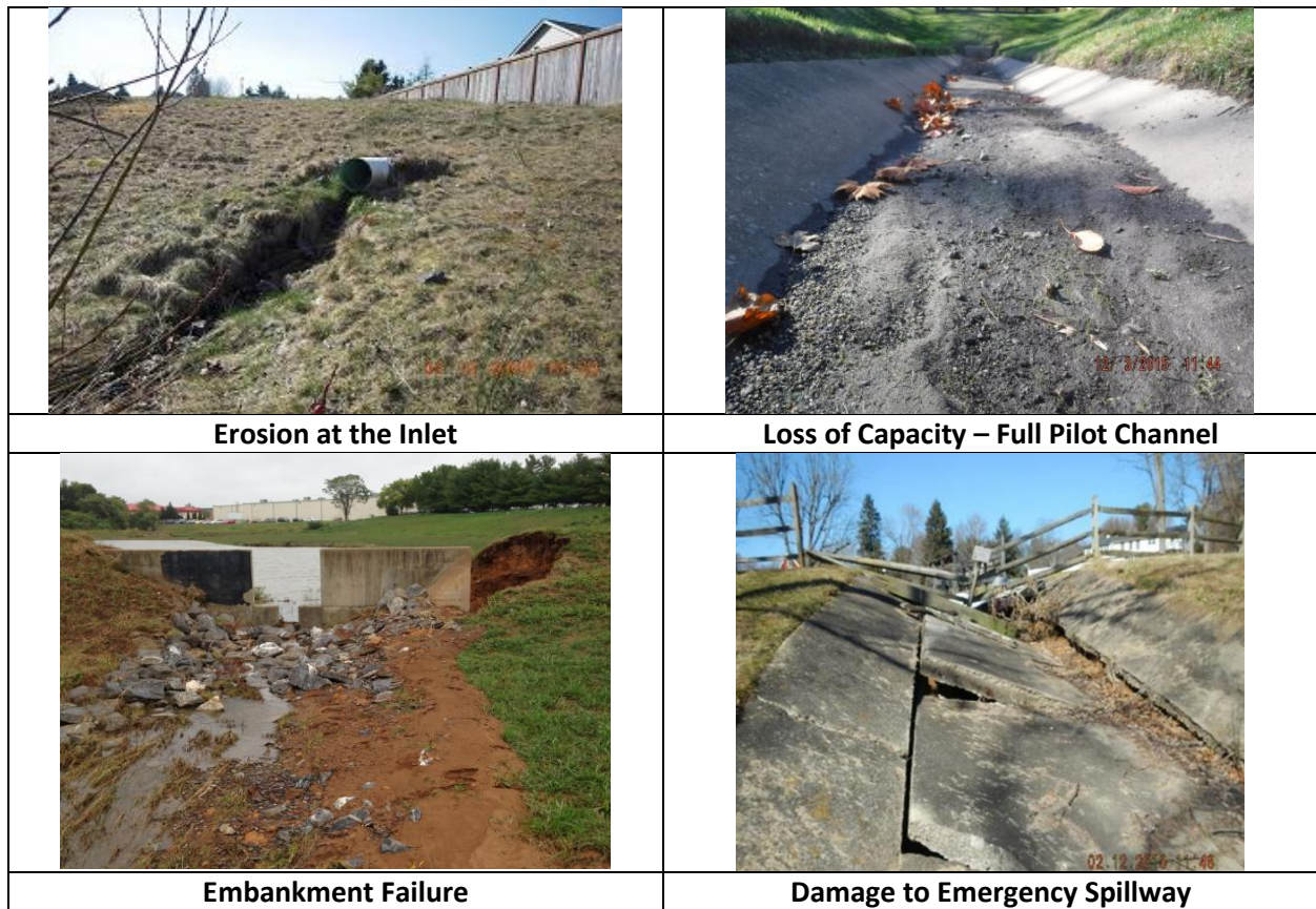
Figure 6. Examples of vulnerable design elements for stormwater ponds.
