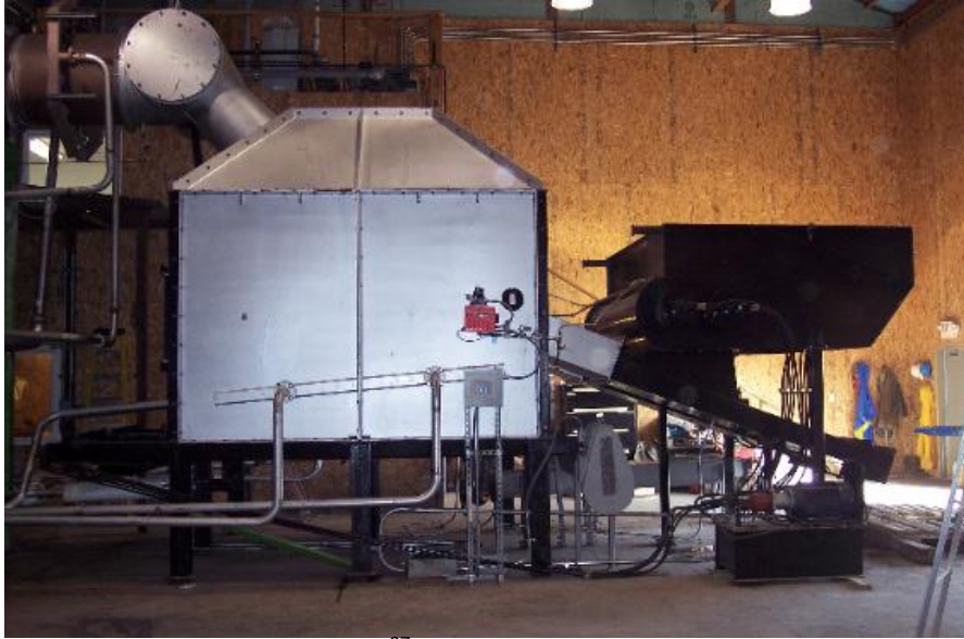
Figure 5. Primary gasifier unit. 97
