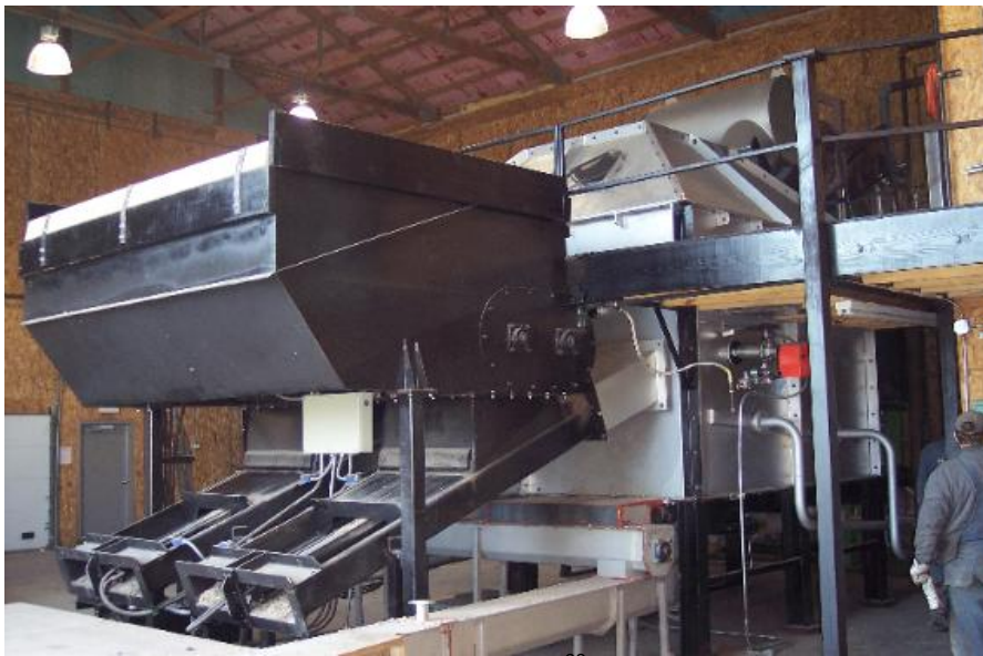
Figure 6. Front of gasifier and feed hopper. 98
