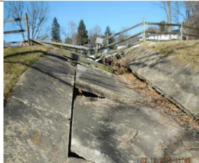
Damage to Emergency Spillway
