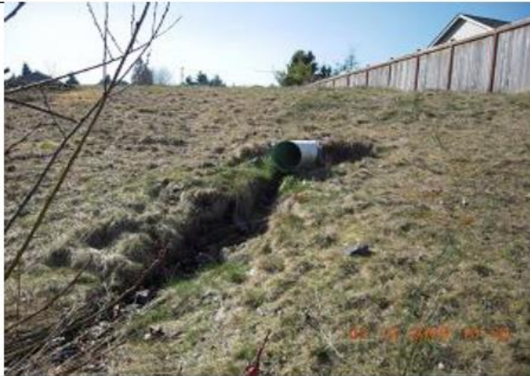
Erosion at the Inlet
