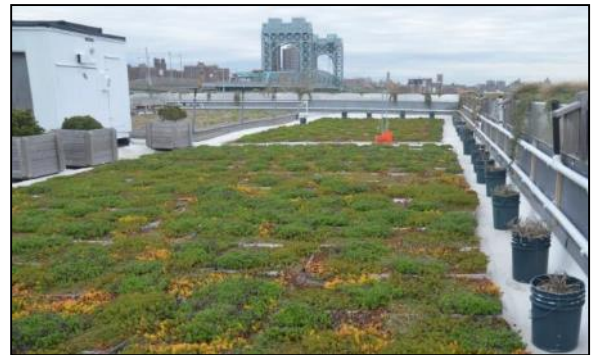
Figure 3 – Typical green roof application (Source: Evan Bindenglass, CBS New York)
