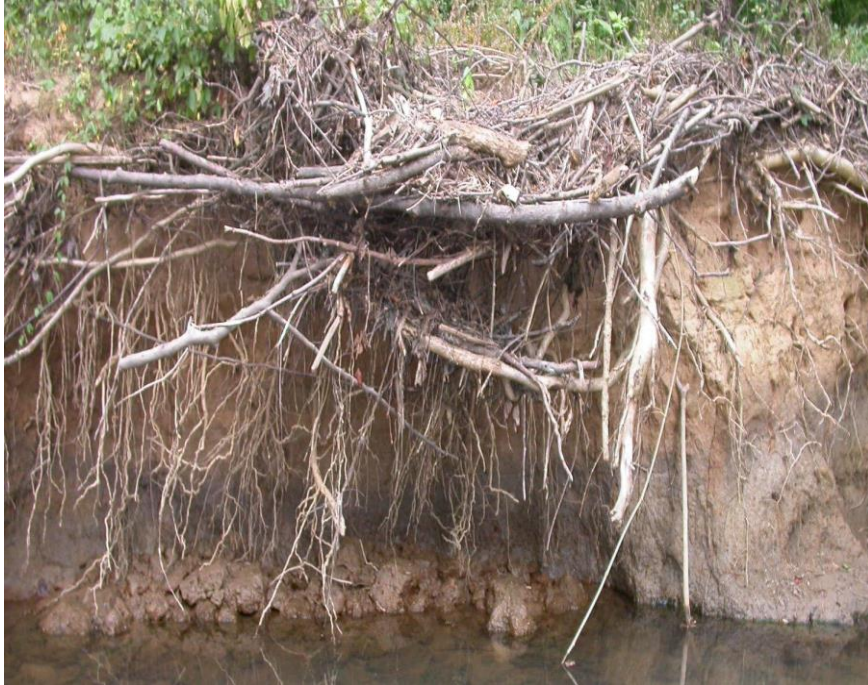
High erosion rates
