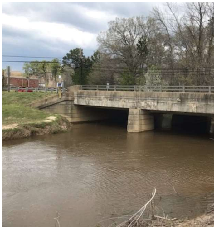
US Geological Survey Weather Gage installed on a bridge over McIntosh Run, St. Mary's County, MD. Photo provided by Eric Colvin.
