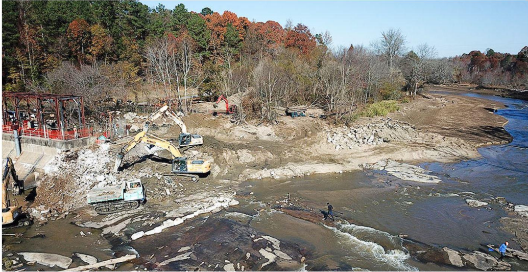
An environmental mitigation firm, Restoration Systems, tearing down the Milburne Dam on the Neuse River outside Raleigh, N.C. The company will turn a profit on the credits it sells from the removal, and advocates say their model could fund dam removals across the country. Restoration Systems
